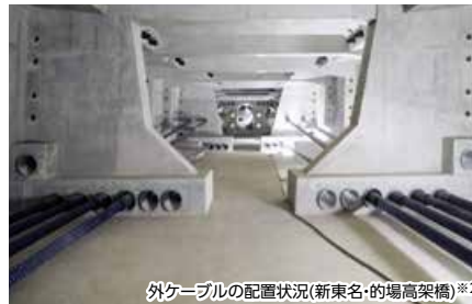
外ケーブルの配置状況(新東名・的場高架橋)※2 Ultra-high strength External Tendons with Epoxy Coated and Filled strands in Matoba Viaduct
